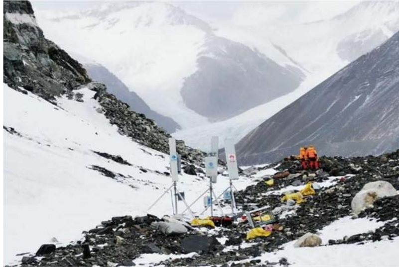
Figure 1.5 Picture of 5G base station deployment at a record high elevation of 6500 m on Mount Everest (after [16]).
